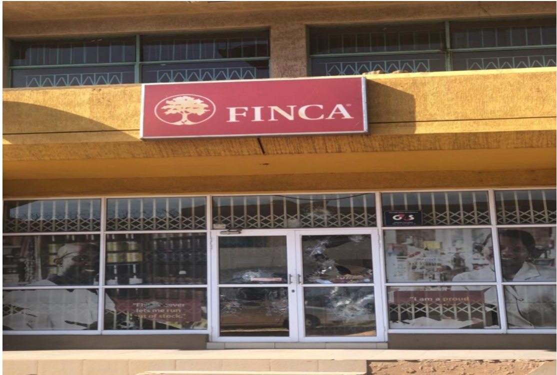
Mkwinda Nyasulu, N. (2019) Broken glass door
